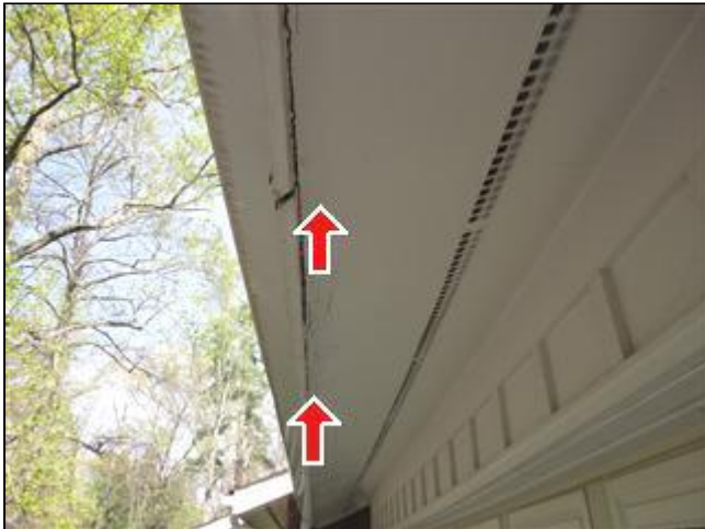
2.5 Item 2(Picture) Soffit damage at garage
