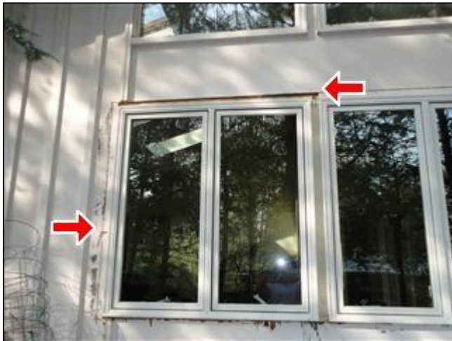
2.0 Item 3(Picture) Damaged siding/trim at front left window
