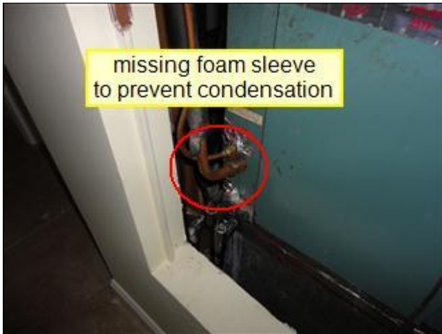
8.7 Item 1(Picture) Missing foam sleeve
