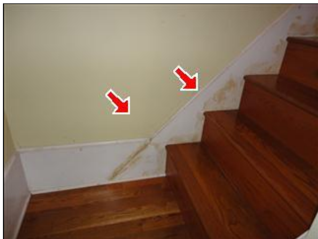
4.3 Item 1(Picture) Unfinished trim at stairs
