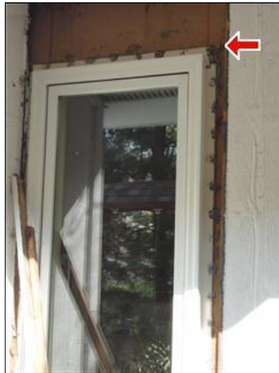
2.0 Item 2(Picture) Missing siding at rear of home
