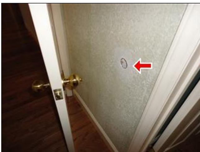
4.1 Item 2(Picture) Guest bedroom drywall damage
