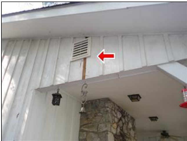
2.0 Item 4(Picture) Damaged siding at left side of home
