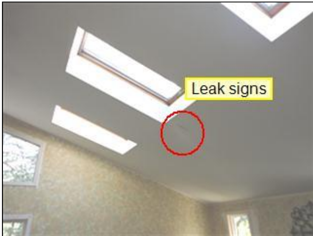
4.0 Item 2(Picture) Leak at ceiling in den
