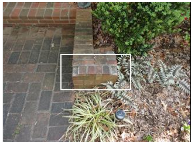
2.4 Item 4(Picture) Missing brick right side
