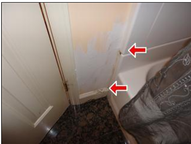
4.1 Item 1(Picture) Guest bath drywall damage
