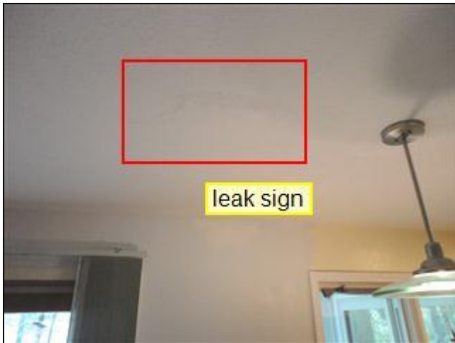
4.0 Item 1(Picture) Leak stain at dining room
