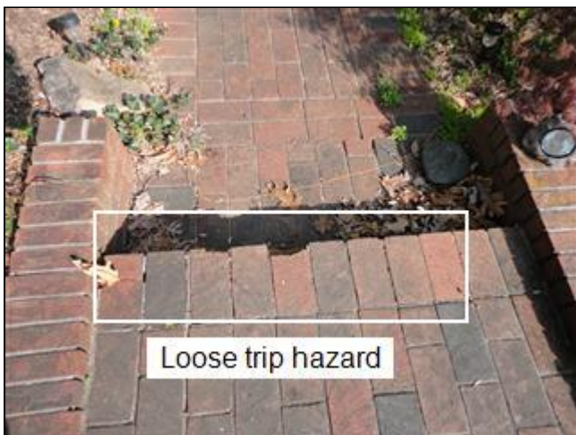
2.4 Item 1(Picture) Loose brick at front walkway
