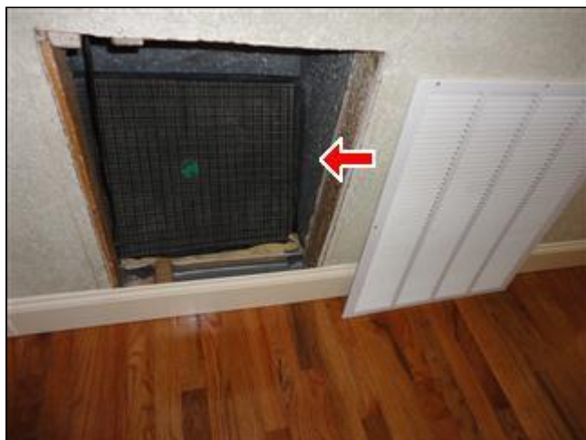
8.3 Item 1(Picture) Dirty filter in hall
