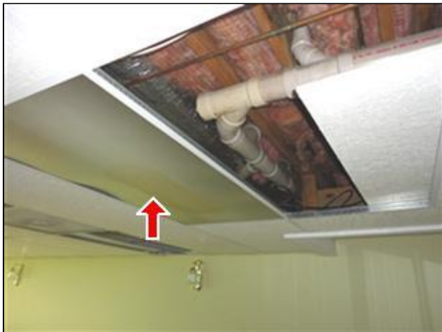
4.0 Item 3(Picture) Basement light panel leak stain
