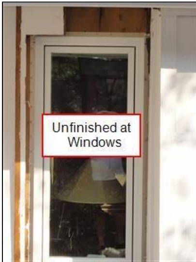
2.0 Item 1(Picture) Missing siding at right side of home
