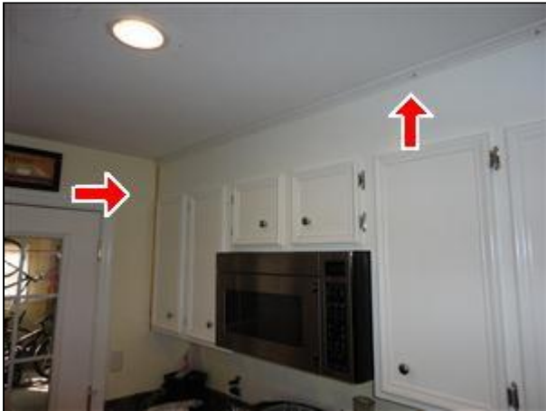
4.4 Item 2(Picture) Trim missing at kitchen upper cabinets
