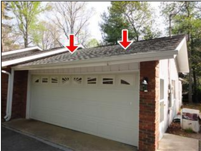
1.0 Item 1(Picture) Improper Shingle Installation
