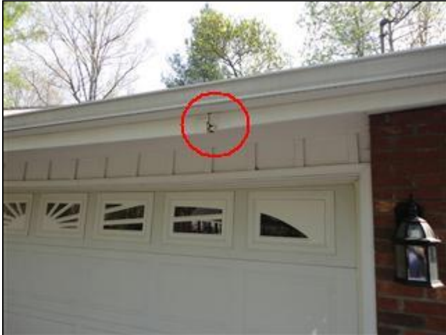
2.5 Item 1(Picture) Fascia deteriorated at garage
