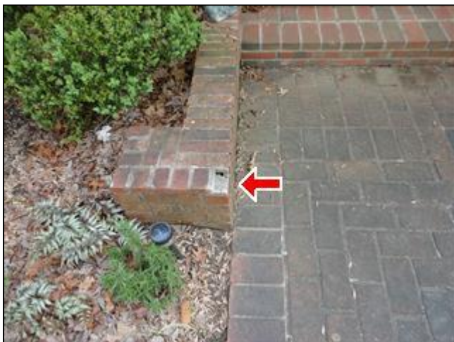
2.4 Item 3(Picture) Missing brick left side
